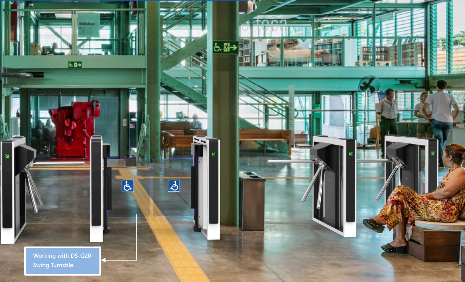
3 lanes DS-Q10 and DS-Q20 disabled lane installed at office
